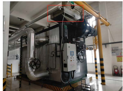
Boiler Heat Recovery Equipment 鍋爐餘熱回收設備
