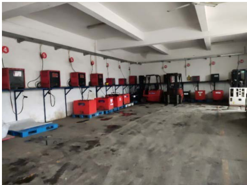
Forklift Charging Idle 叉車充電間
