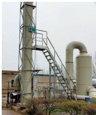
Sewage Treatment Equipment 污水處理設備
